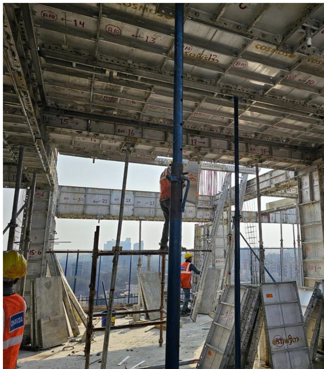
Equipment name : Aluminum Monolithic Formwork Country of origin : Malaysia Amount invested : ₹37.6 crores 1
